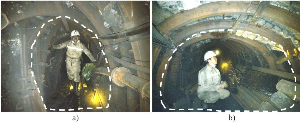
Fig. 6. The roadway is deformed when the coal pillar width is 15–20 m at Khe Cham coal mine.
