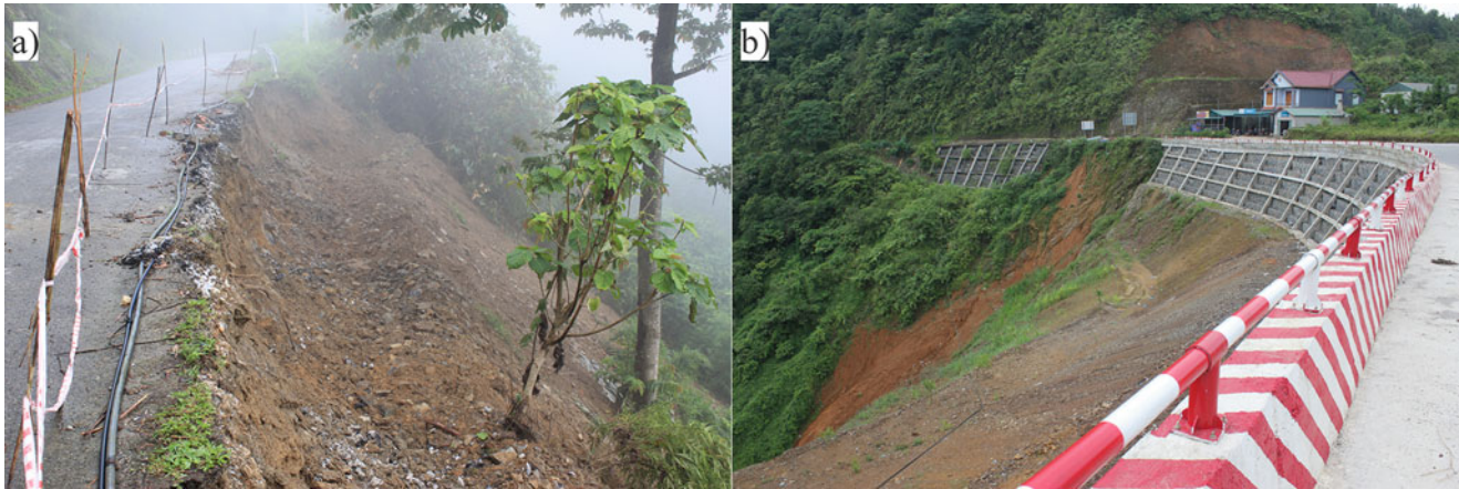
Fig. 2 Landslides at the national highway 34 km 192 + 500 (a), and at Km 200 + 300 (b). Photo by T. K. Nguyen
