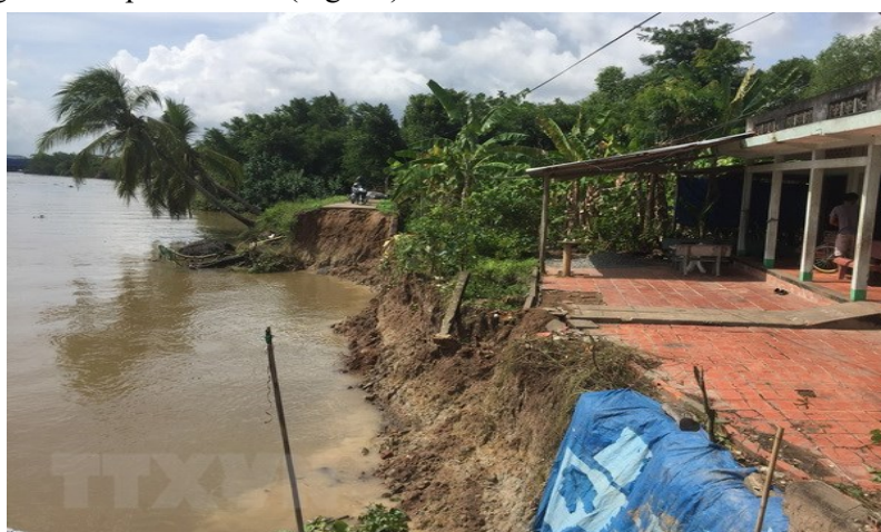
Fig. 11. The riverbank erosion in My Duc Dong, Cai Be District (2021)
