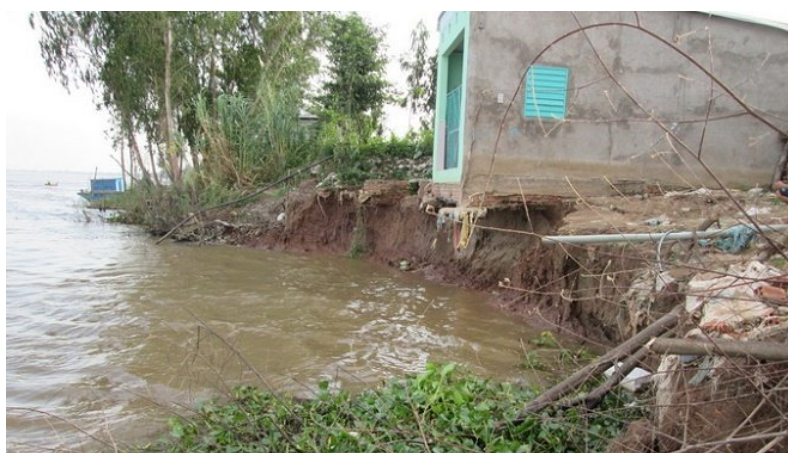
Fig.12. The riverbank erosion caused by boat activities (2021)
