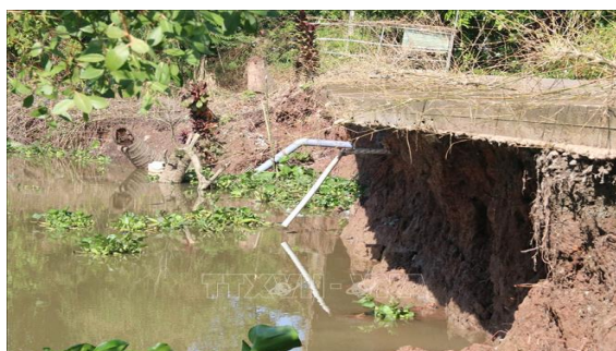
Fig. 9. Landslide creating a cleft deep into roadbed 54C (2022)
