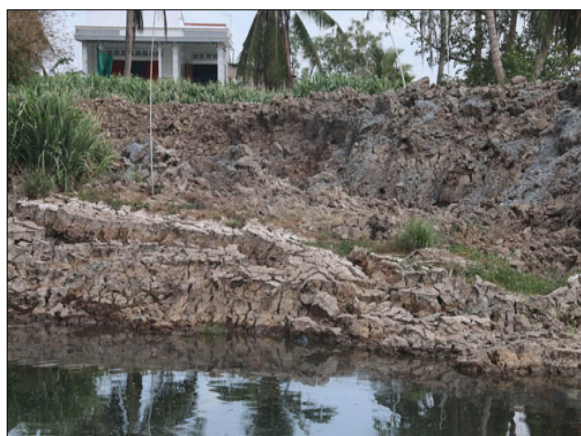
Fig.14. Canal bank erosion due to weak geology (2020)
