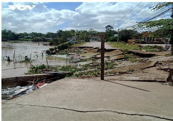
Fig.16. Some landslide recovery works in Tien Giang completed in a short time have subsided.
