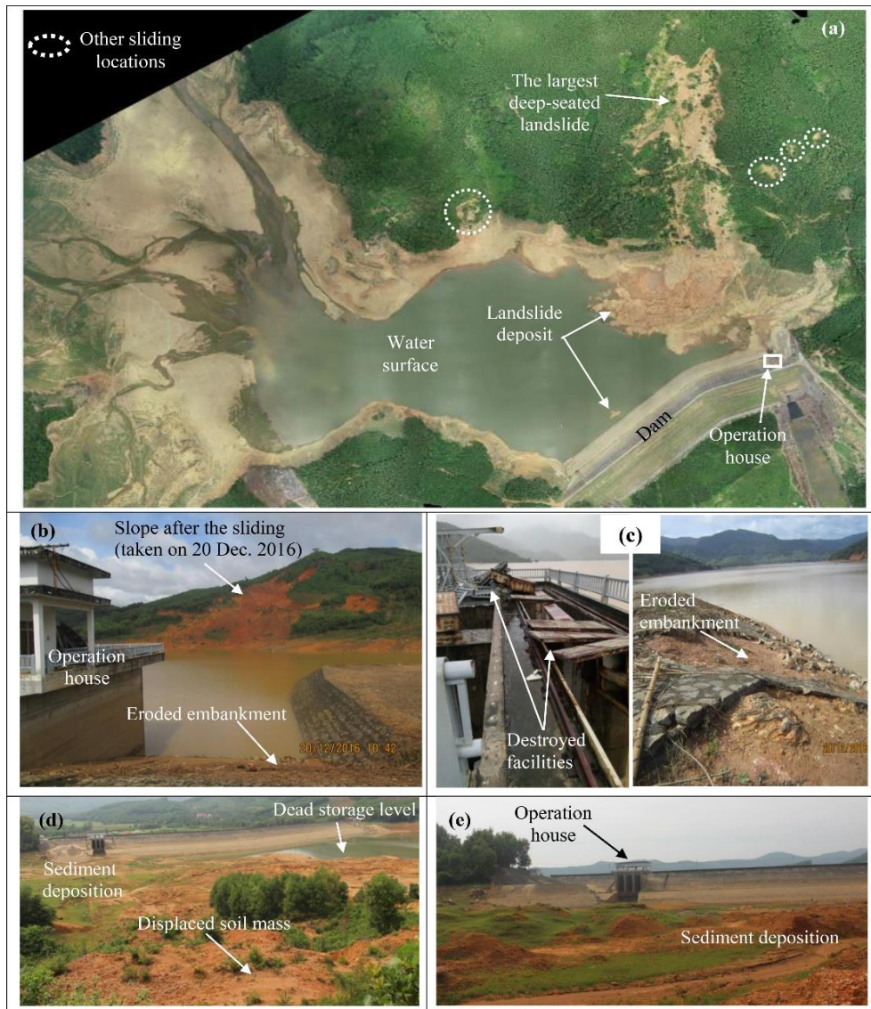
Figure 2. (a) UAV's photo of the Van Hoi reservoir, (b, c) Photo of the slope after sliding and its extensive damage to the dam facilities on December 20, 2016 (Photos courtesy by Do Canh Hao), and (d, e) Sediment deposition reservoir floor took on October 4, 2019
