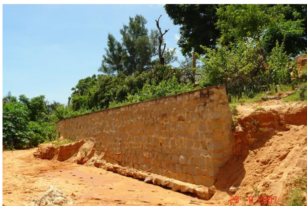
Figure 2. The protective structure was destroyed after the rains
