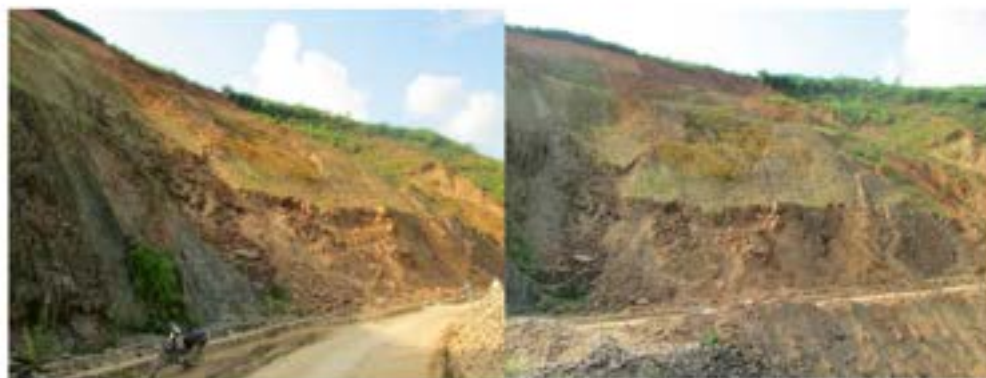
Figure 2. Two photos of the landslide on the slope wall of National Road 279, near the right bank of Nam Kim stream, Na Pa village, Muong Kim commune, Than Uyen district. Source: Vietnam Institute of Geosciences and Mineral Resources.
