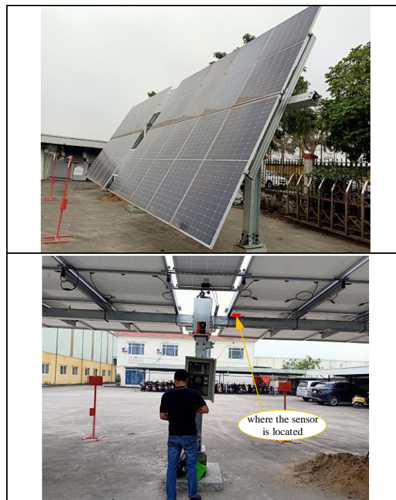
Figure 36. The MPU6050 sensor is fixed on the test solar tracking system
