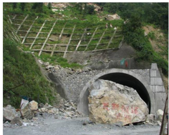
Figure 3. Rock fall at the Longxi tunnel portal from a high and steep slope (Tianbin, 2012).
