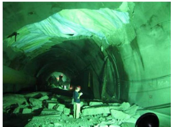
Figure 2. Collapse of the tunnel roof of secondary lining concrete in the Longxi tunnel (Tianbin, 2012).
