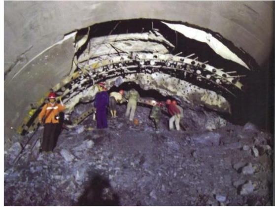
Figure 1. Collapse of the tunnel at the crossing of the fault (Tianbin, 2012).
