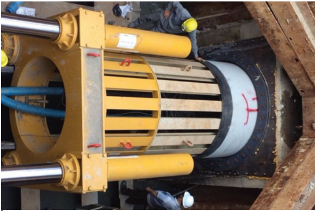
Figure 4. Pipejacking a pipeline D1500mm cross Nguyen Van Linh road, Binh Chanh district, Hochiminh city (Baogiaothong, 2018)
