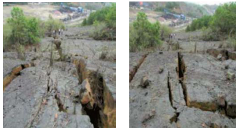
Fig. 2. Joints and cracks along the surface of the actual slope
