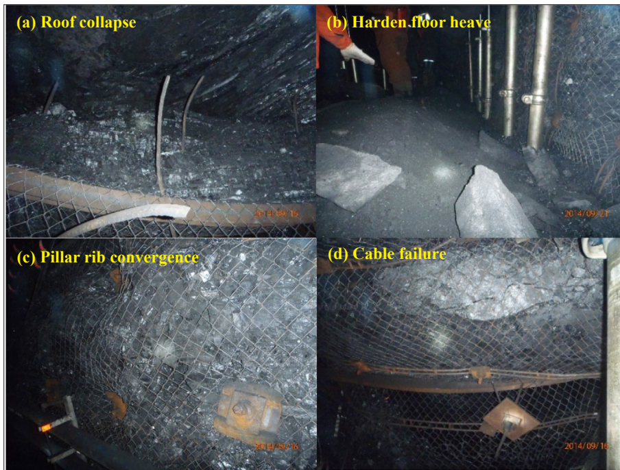
Fig. 2. Deformation characteristics of 3905 headgate due to retreating Panel 3805.
