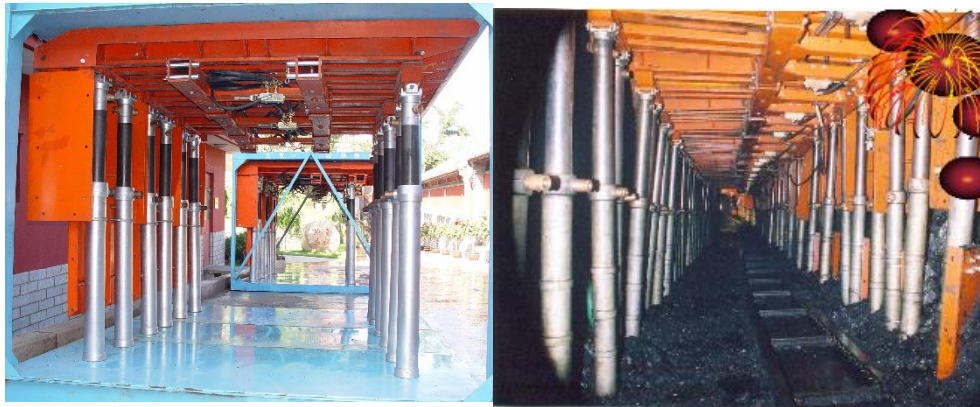
Fig. 2. (a) Semi-mechanised support ZH-1600 at surface and in underground [5].
