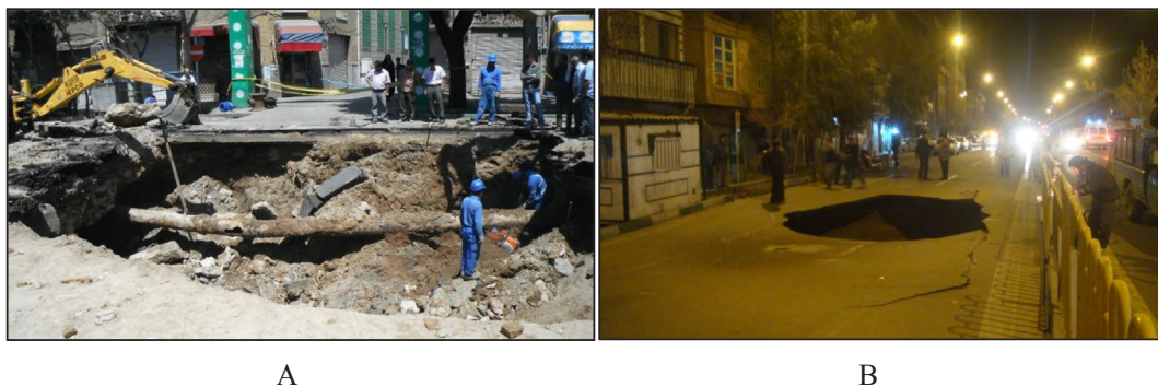
Fig. 8. Collapses in Molavi Street, nearly chainage 4 + 100.
