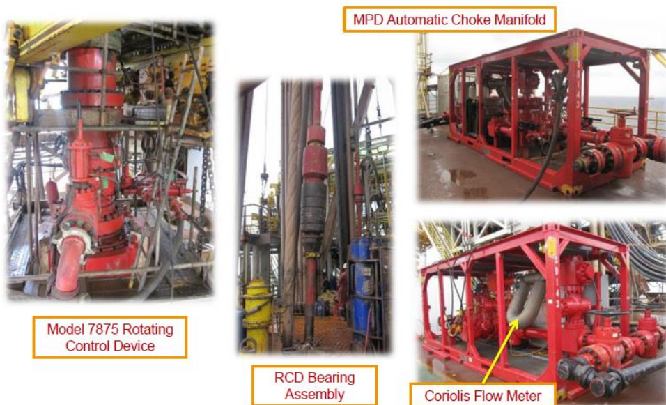
Figure 2. MPD key equipment in use at Bien Dong POC
