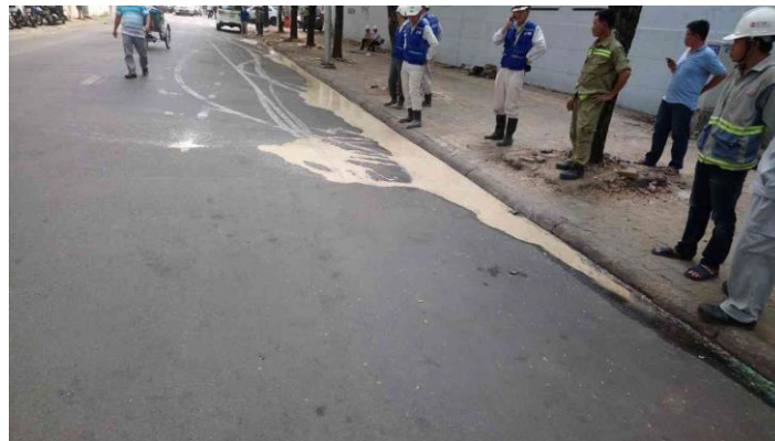
Figure 5. Support fluid was spouted on the street when blow-out occurred
