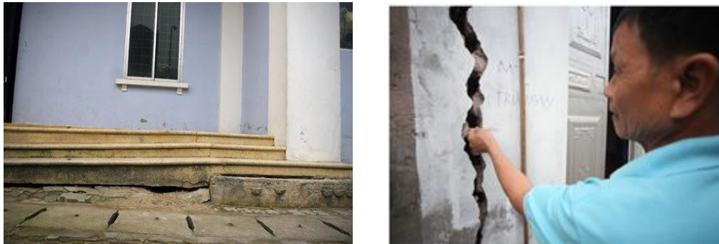
Figure 2. Damage to structures due to land subsidence in Hanoi
