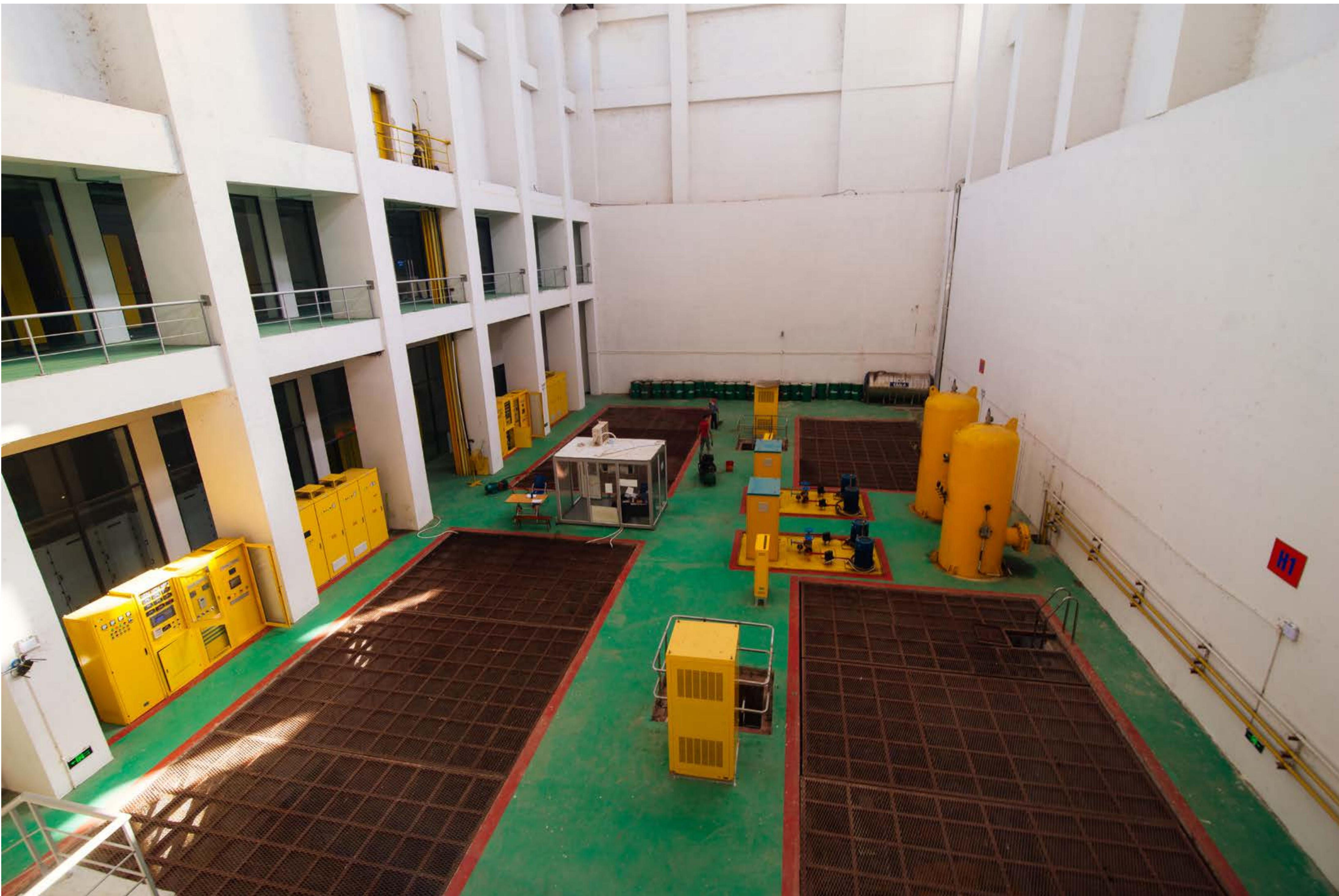
Photo: Inside the Cam Thuy Hydropower Plant 1
