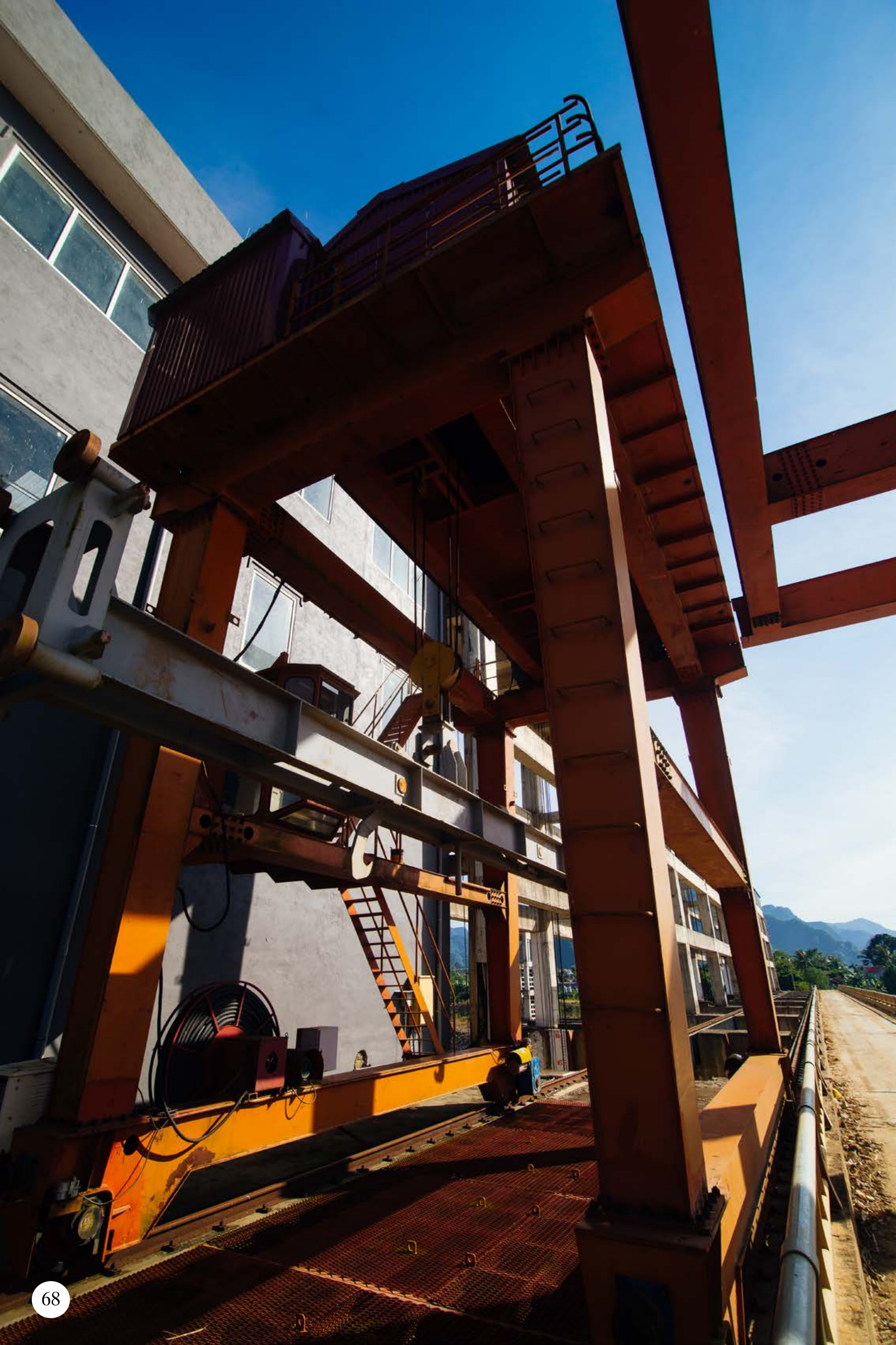
Intake gate of Cam Thuy I Hydropower Plant
