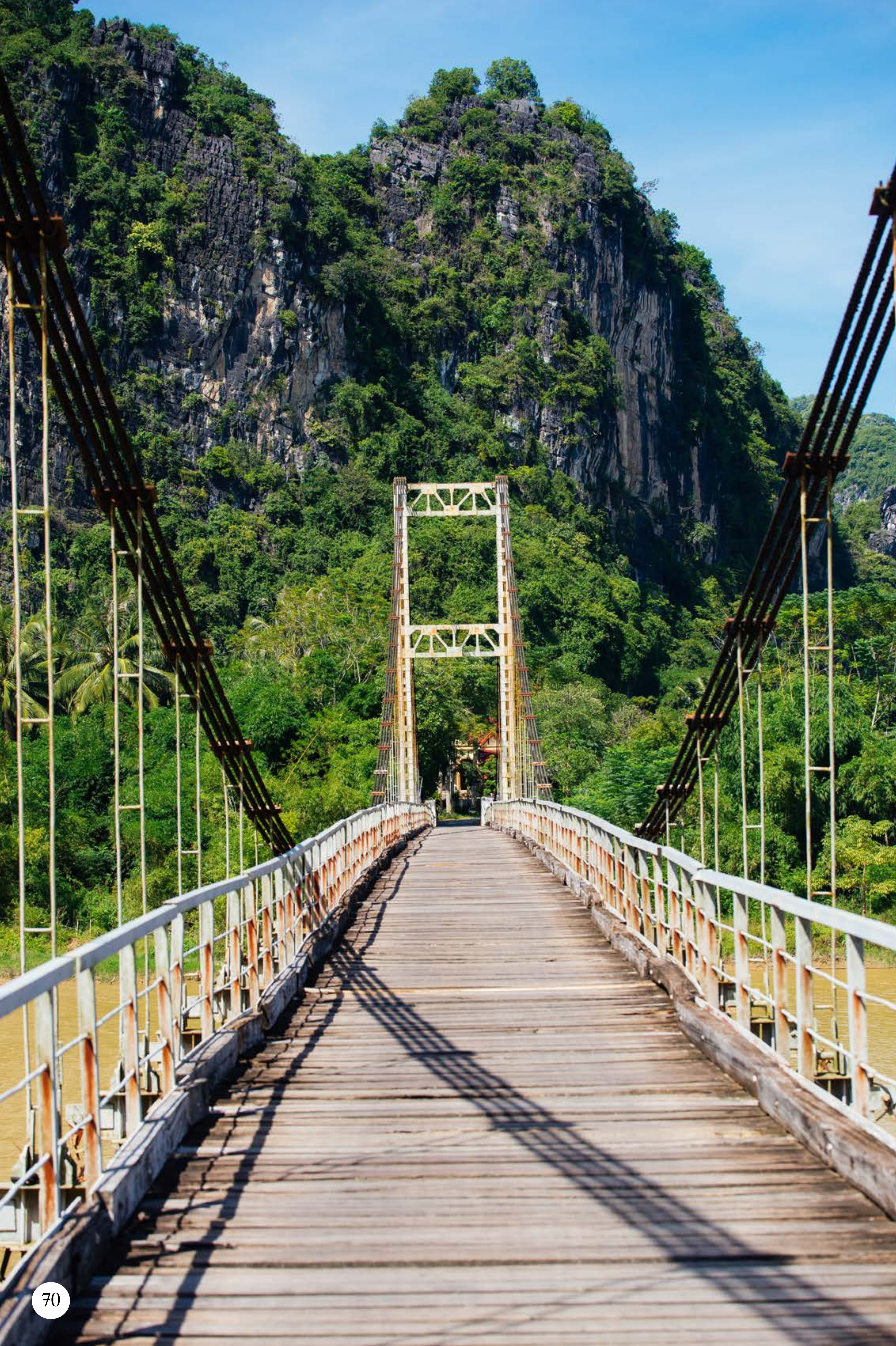
Cam Thanh sus- pension bridge con- necting the Cam Thanh and Cam
