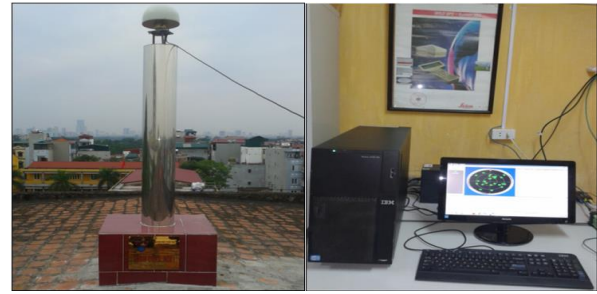
Fig.7. Installation of CORS N001 station system at Hanoi University of Mining and Geology
